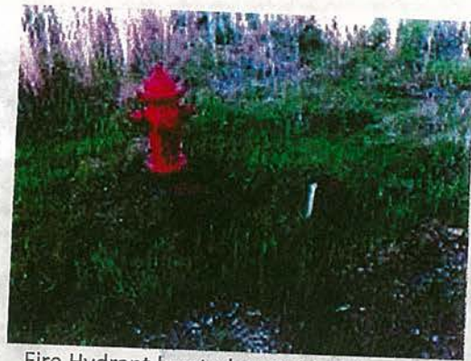
Fire Hydrant located on Subject Property
